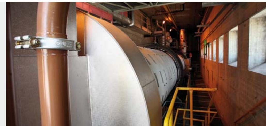
Erzo Oftringen sewage treatment plant (Switzerland): rotary kiln for the incineration of sewage sludge
