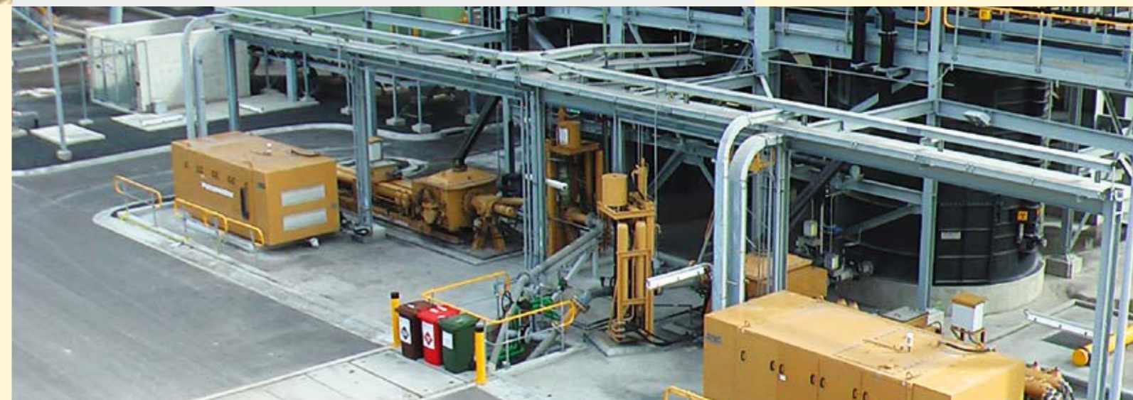
A KOS 25100 pump installation (Kogan Creek, Australia) for fly and bottom ash
