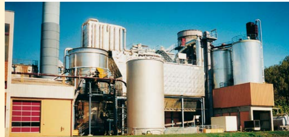
Sewage sludge reception station consisting of reception and storage silos: Incineration of foreign sludge at the main wastewater treatment plant of Stuttgart-Mühlhausen
