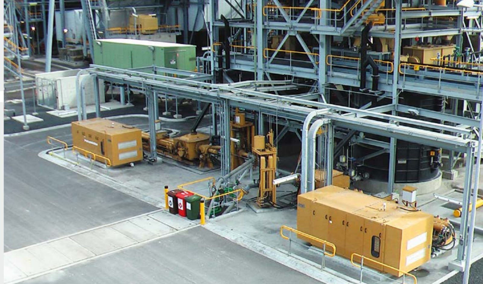
Redundant transport of fly and bottom ash from a power plant
